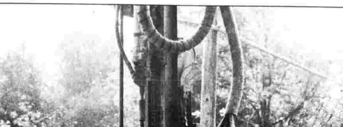
POWER DRILL — Doug Schumann Sr., right, and Doug Schumann Jr., owners of D&H Drilling & Blasting, drill holes in Keeney Street for blasting. The Schumanns, subcontractors for Glenn Construction Co., are working on the Keeney Street sewer project.
